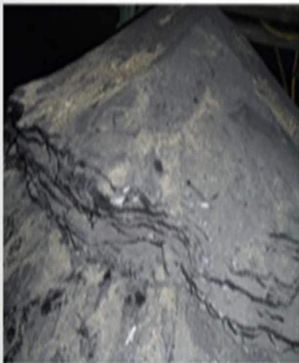
Deposits on Riser Termination Device
